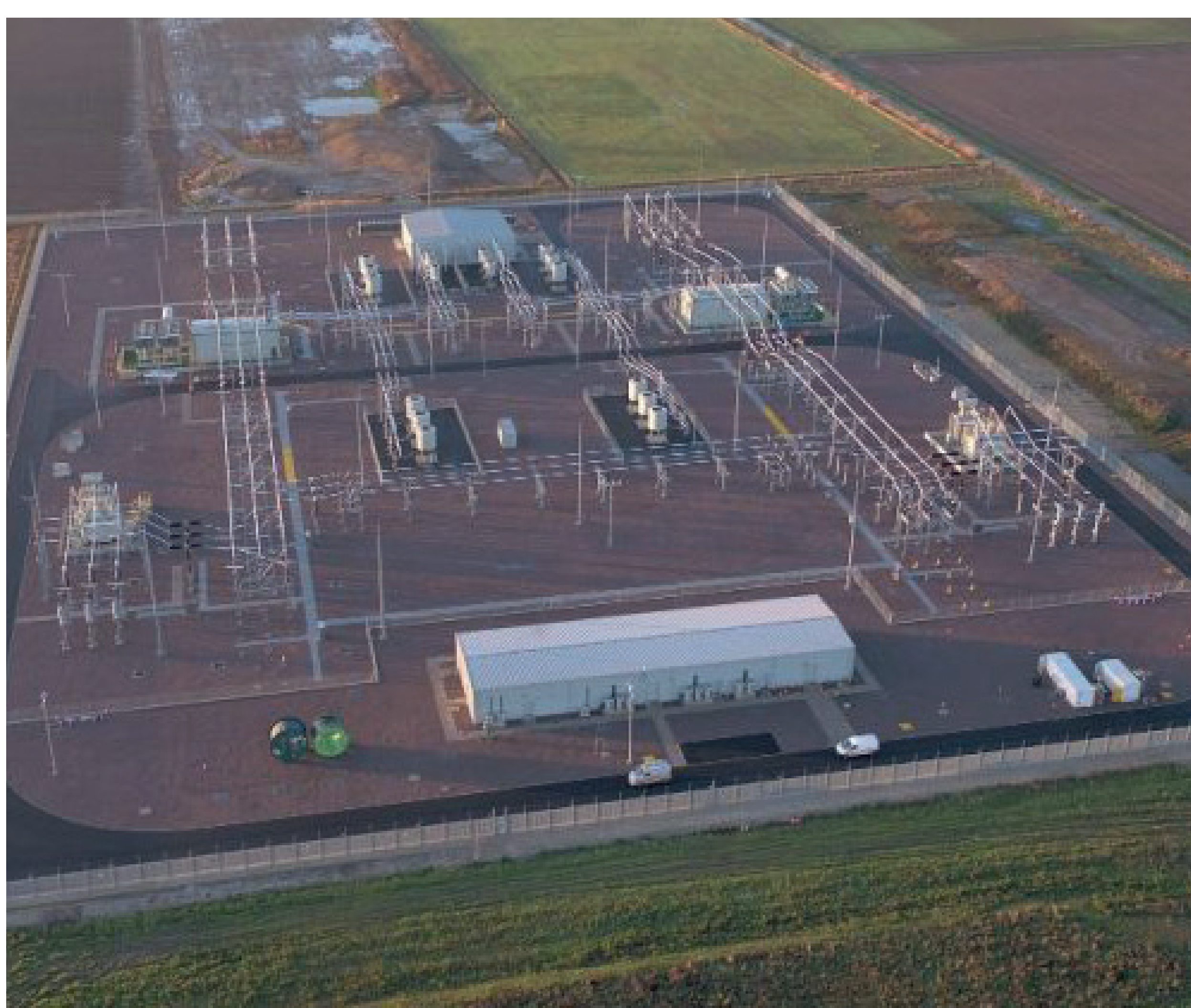
Substation with Air Insulated Switchgear (Triton Knoll, Lincolnshire)
